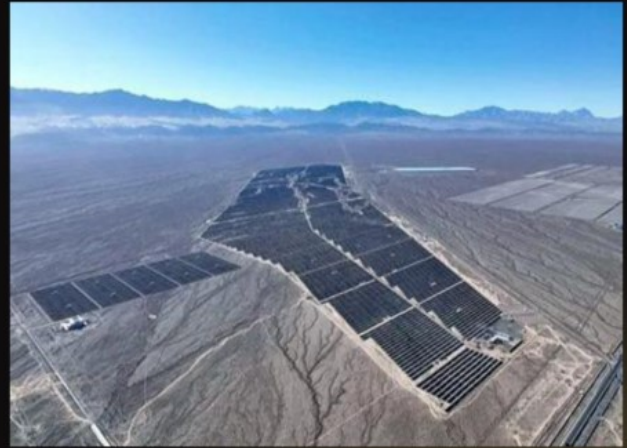
Yumen Oilfield Photovoltaic Project
