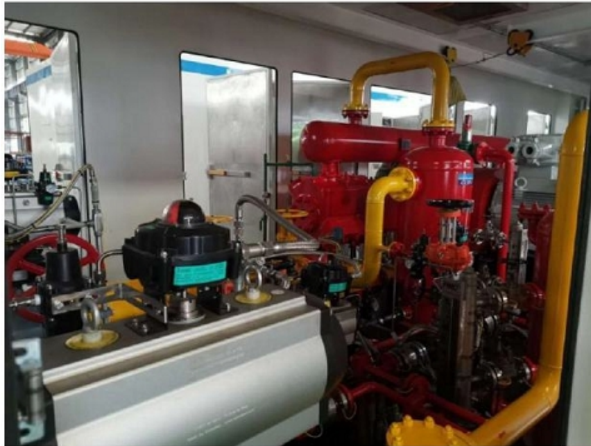
Our negative pressure compressor unit.
