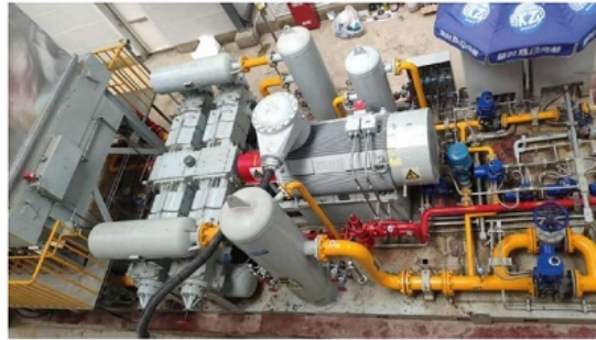
Our gas transmission compressor unit.
