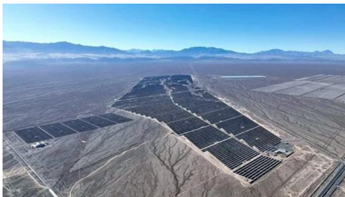
Yumen Oilfield Photovoltaic Project.
