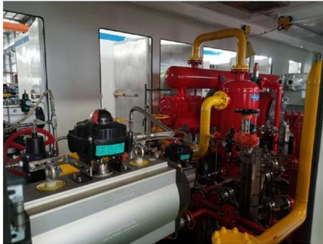
Our negative pressure compressor unit.
