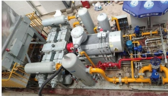
Our gas transmission compressor unit.
