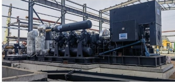
Our ultra-high pressure gas injection compressor unit.
