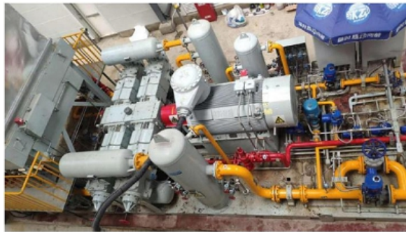
Our gas transmission compressor unit.
