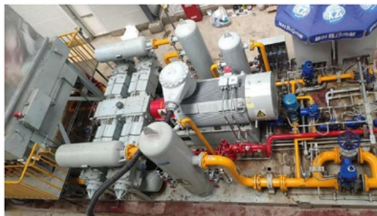
Our gas transmission compressor unit.
