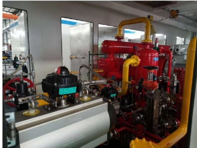
Our negative pressure compressor unit.
