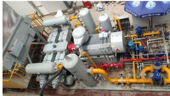
Our gas transmission compressor unit.
