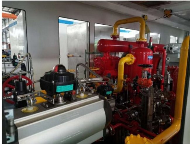
Our negative pressure compressor unit.
